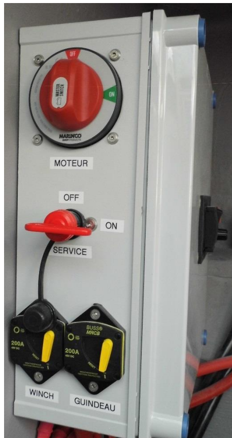
Winch and windlass circuit breaker
